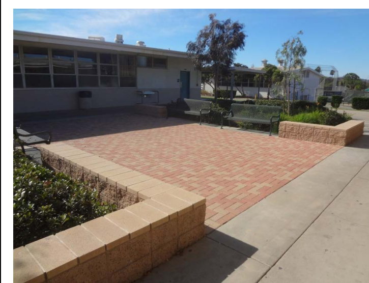
Photo -4 Curb Appeal – Courtyards The courtyards between the classrooms have been recently upgraded with masonry planter walls, benches and pavers.
