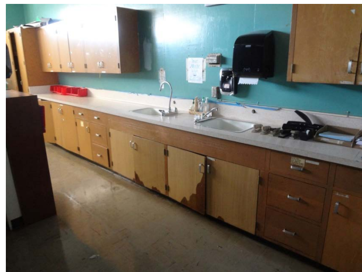
Photo -5 Classrooms The finishes in the classrooms show significant wear and tear. The sink does not meet accessibility requirement.
