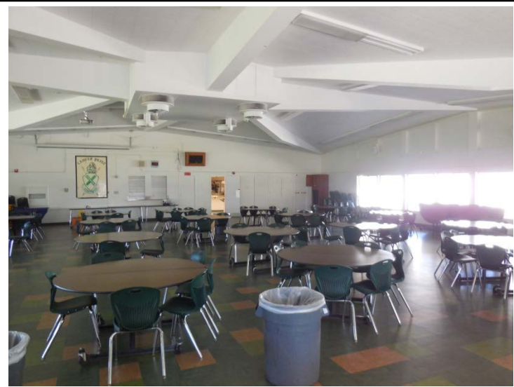
Photo -13 Cafeteria / MPR The cafeteria doubles as the campus MPR. There is no air conditioning and the finishes are dated. The windows lack shading and have been painted to reduce glare and heat.
