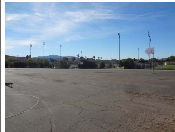
Photo -7 Black Top The basketball court surfaces has extensive cracks and the striping are heavily faded.
