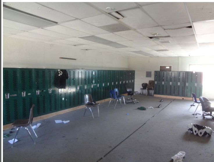
Photo -6 Football Locker Rooms The football player locker rooms are in portable buildings. Finishes are in poor conditions and ventilation may be insufficient.
