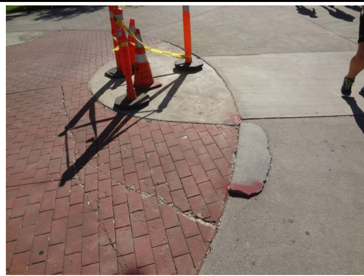
Photo -1 Concrete and Site Work Issues Throughout the site there are cracked concrete pavers and concrete surfaces.
