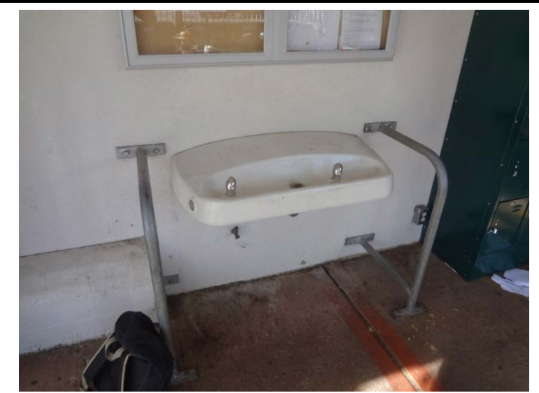
Photo -4 Accessibility Upgrades Throughout the site there are accessibility compliance issues.
