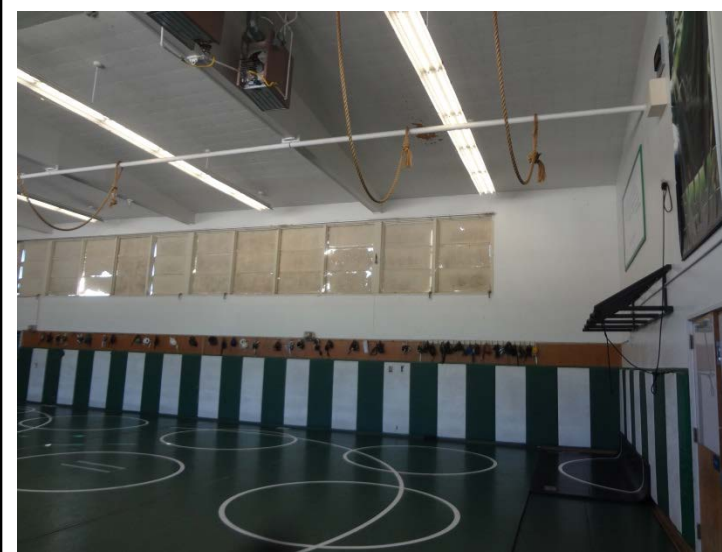
Photo -11 Activity Rooms The activity rooms have not been upgraded. The HVAC does not function properly. The windows lack shading and have been painted to reduce glare and heat.
