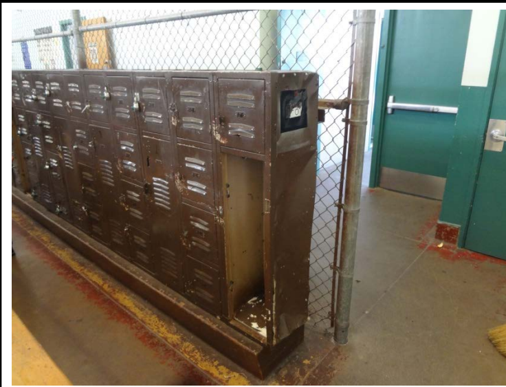
Photo -3 Locker Rooms The locker rooms are in poor condition. Several lockers have been damaged.
