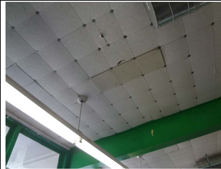
Photo -15 Classroom Ceilings The condition of the ceiling tiles is poor and mechanical fasteners have been added to hold the tiles in place in expense of the appearance
