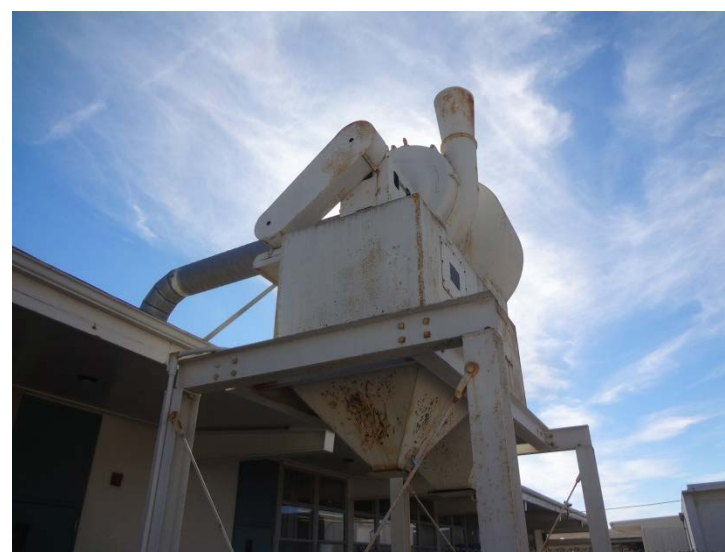
Photo -10 Dust Collector The dust collector may require major service or replacement.
