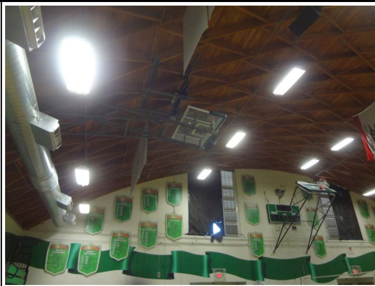
Photo -2 Gym The gym currently has no HVAC. The acoustic tiles were removed and it now has a reverberation issue. The sport flooring also shows signs of aging.
