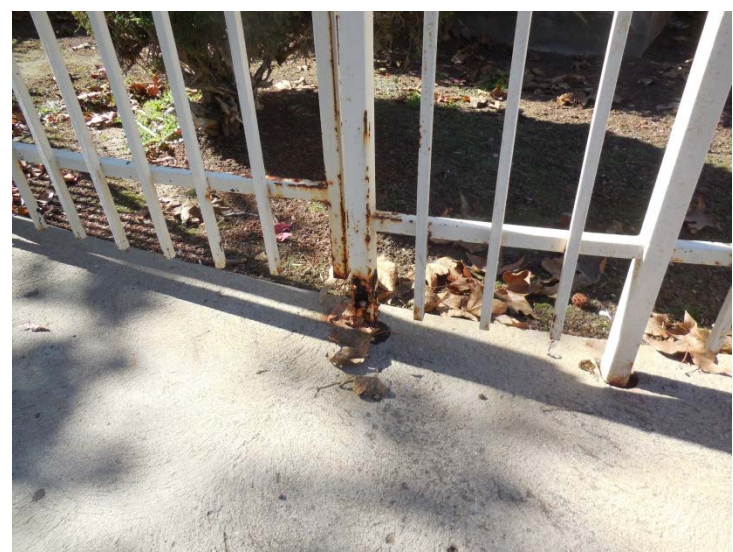
Photo -9 Fencing The fencing throughout campus shows extensive rust and water damages.
