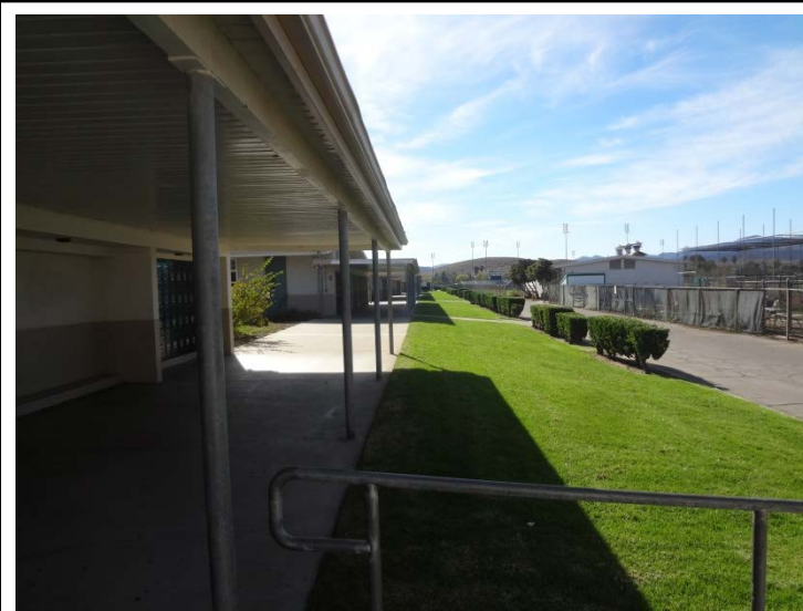
Photo -6 Curb Appeal – Covered Walkways The covered walkways extend to the rear of the classroom buildings, providing shade to the locker area as well as shelter from the rain.
