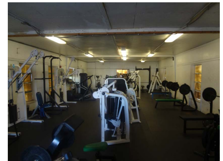
Photo -8 Sports Weight Room Currently the weight room for all other sports besides football is located in a large temporary structure that has insufficient ventilation, lighting and thermal insulation.
