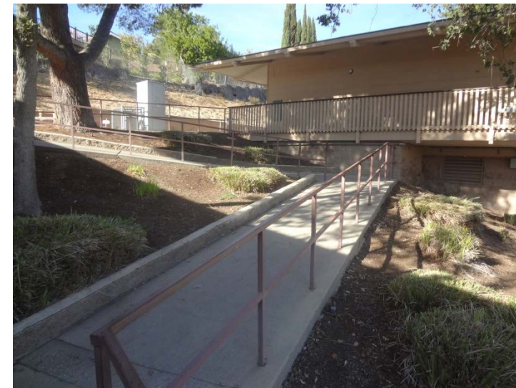
Photo -7 Ramp to Second Floor Ramps on campus are not current with accessibility standards which is an issue for fire egress as well
