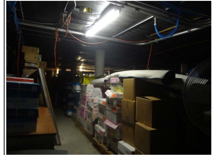
Photo -4 Storage Under Building The storage area underneath the southern most building is large and may require fire life and safety related upgrades.
