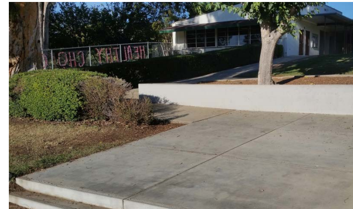
Photo -3 Stairs and adjacent slopes do not appear to comply with current accessibility standards.
