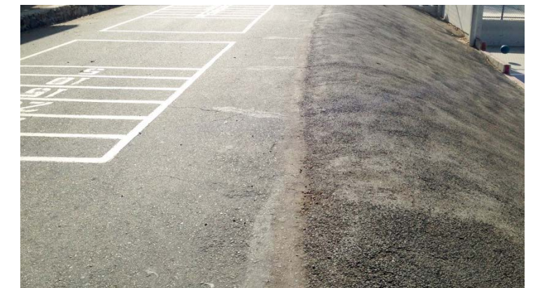
Photo -6 Steeply sloping asphalt adjacent to play areas is an accessibility and safety concern.
