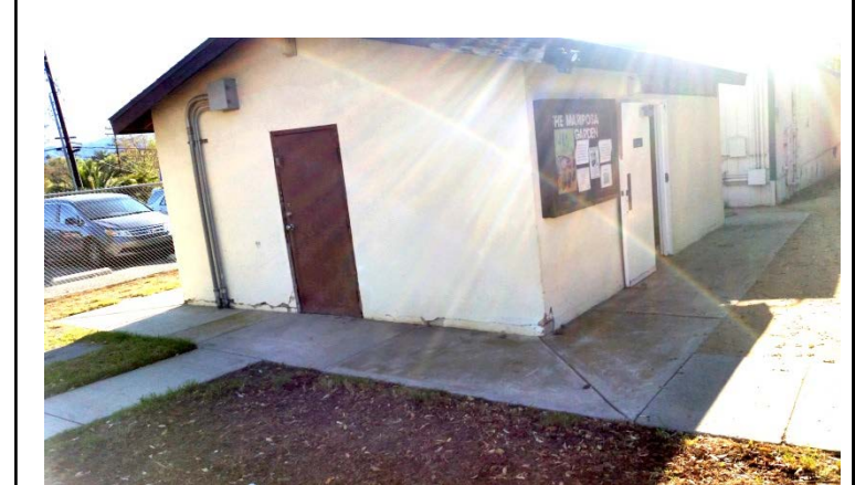
Photo 8 Building Name: Restroom Building Number: 6 Description: Building does not meet accessibility requirements. Additionally, there is no accessible path of travel from the upper campus to this location.
