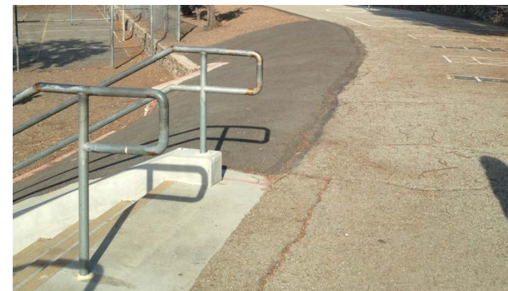
Photo -5 Steeply sloping asphalt adjacent to play areas is an accessibility and safety concern.
