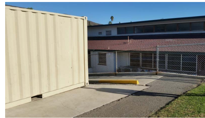
Photo -1 Landing at top of ramp does not appear to comply with current accessibility standards
