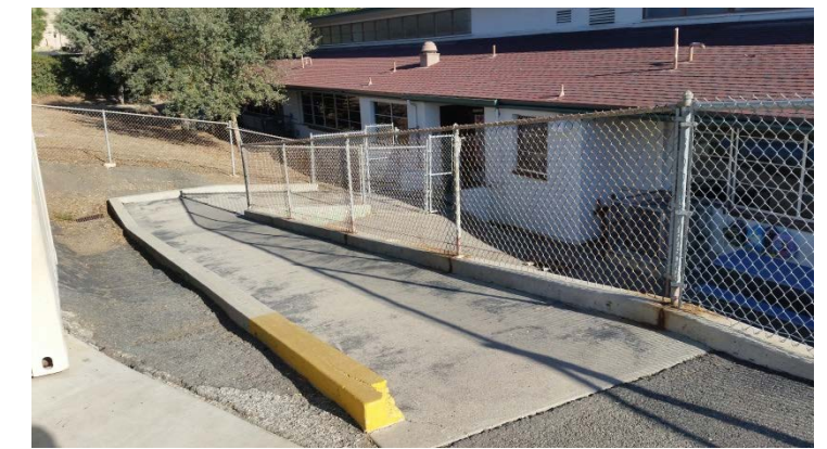
Photo -2 Ramp does not appear to comply with current accessibility standards.
