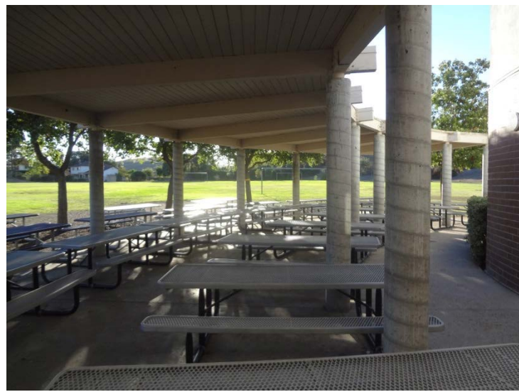
Photo -17 Building 2: Shade Structure Concrete columns with wood rafters. In good condition and sufficient to supply needs of campus
