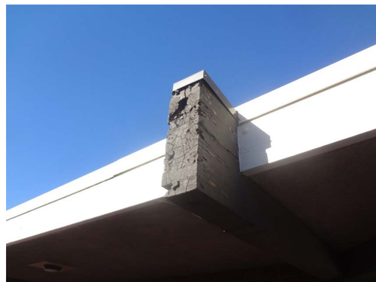
Photo -5 Building 1 Typical wood rafter, condition throughout campus varies some are in need of repair
