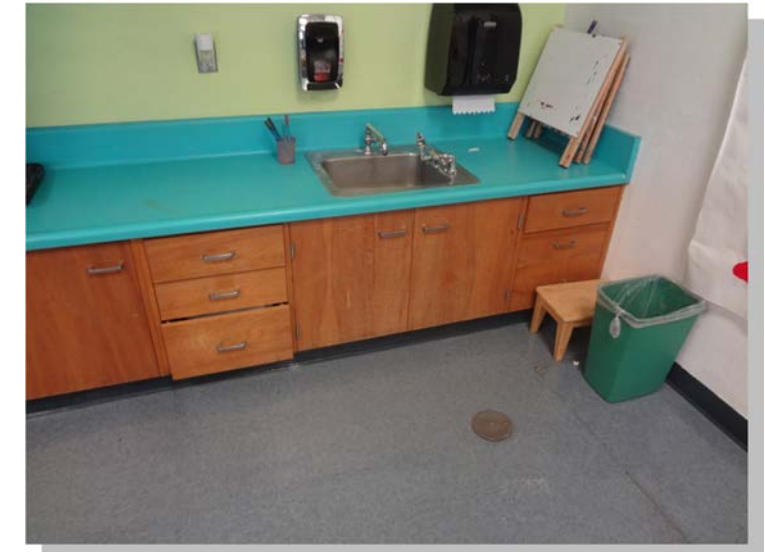
Photo -2 Classroom sinks have not been made to comply with current accessibility standards with exception of the kindergarten classrooms
