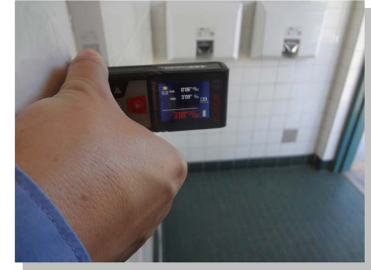
Photo -5 While the bathrooms have been upgraded for accessibility, they do not have the required clearance at the entry to meet current accessibility standards
