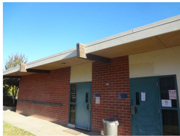
Photo -1 Building 4 Typical building façade with brick/masonry structural system supporting large rafters that cantilever out over walkway
