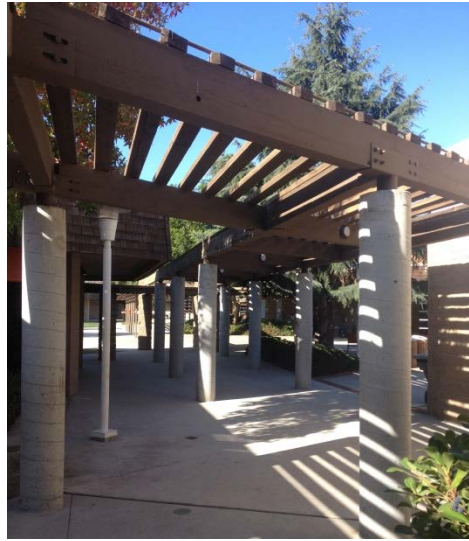
Photo 9 Building Name: Lunch shelter Building Number: N/A Walkway from lunch shelter area.
