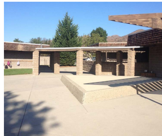
Photo 3- The exterior assembly/stage are potential trip hazard.
